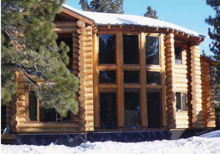
Above: The log shell consists of courses of western red cedar logs, known for their insulation properties. Top Right: A contractor checks the specs of the home during a construction break.
